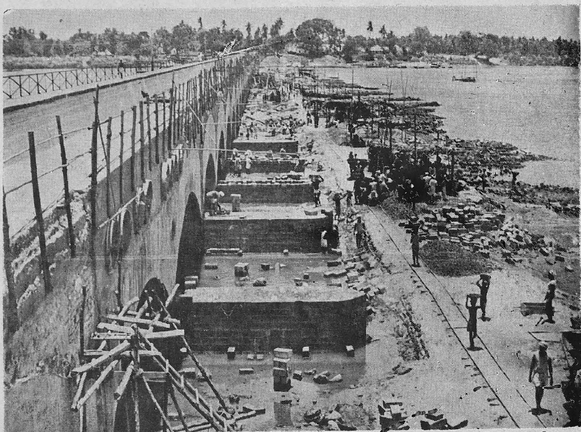
PORTION TO EAST OR LEFT OF RECONSTRUCTION AREA VIEWED FROM RECONSTRUCTED ROAD SLAB
