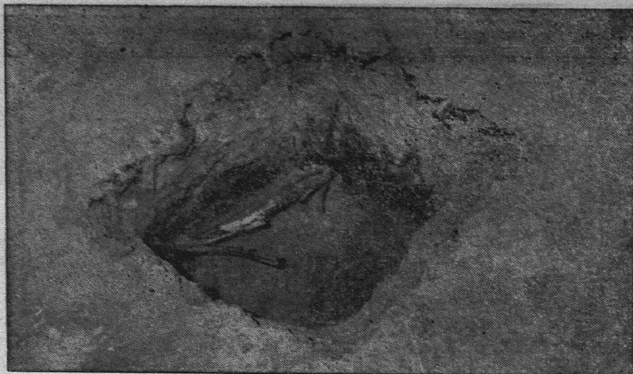
Fig. 2.5.3. A closeview of the pit in the distressed site showing the tree roots in the subgrade.
